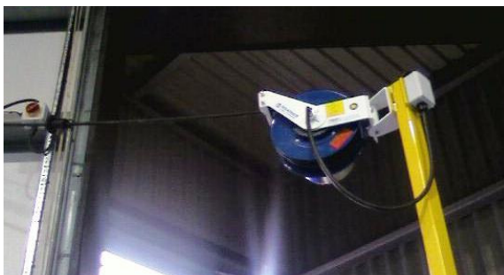
Cable Reel Drum
